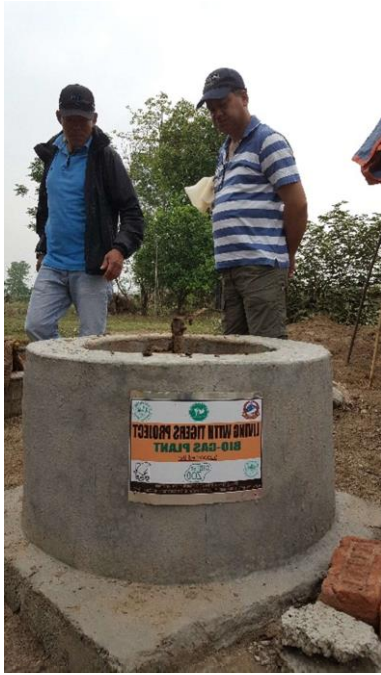
Photo 4: Biogas plant installed in Kalabanjar UC, CNP
